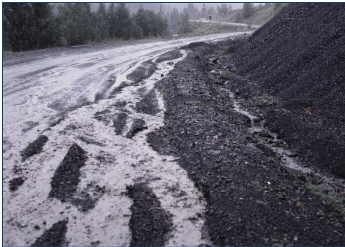
Figure 5. Haul road runoff on a road located in highly-erosive Mancos Shale. The ditch has filled with eroding material and failed, causing water to run down the road.
