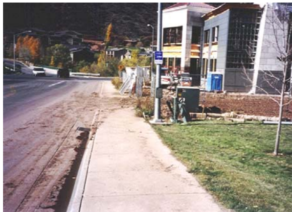
Figure 26: Construction sites can be the source of sediment that is carried into storm drains and discharged into the rivers. A “vehicle tracking pad” composed of washed gravel would act as a floor mat for vehicles and help to contain mud within this construction site.
