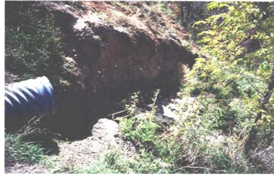
Figure 12: Many of the existing storm outfalls into the river shoot water onto the bank, eroding the hillside. Current designs usually incorporate a flared end section and riprap (rock) outfall to dissipate energy of runoff and prevent erosion at the outfall.
