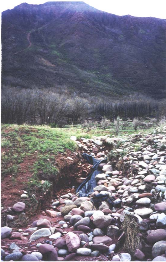
Figure 17: This storm rundown near the Glenwood Municipal Operations Center along Midland Avenue is highly eroded. Improved erosion protection with grouted rock rundown will keep runoff from scouring sediment that often ends up in the river.
