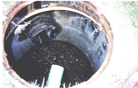
Figure 28: This “dry well” in Cardiff Glen directs stormwater to a holding basin for percolation into the gravel. Maintenance is necessary to remove accumulated sediment. A major storm could overwhelm this system and back-up in the pipe or flow out the manhole cover.
