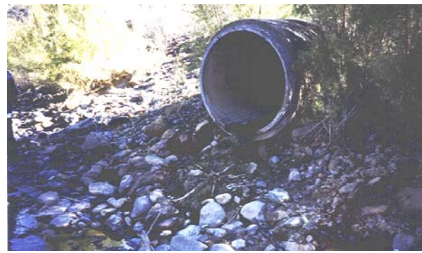
Figure 16: This 48-inch RCP outfall directs runoff from the undeveloped hillsides in the north Glenwood area across I-70 and into the Colorado River.
