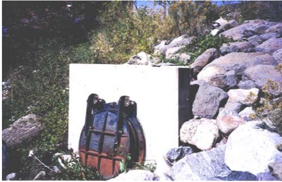
Figure 11: This 30-inch outlet to the Colorado River at the West Glenwood I-70 exit uses a flap gate to prevent river flooding from flowing into the pipe. The outfall is a potential water quality sampling point for highway runoff.
