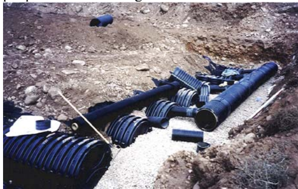
Figure 31: An underground detention site is under construction in Glenwood at this development site. Underground systems are difficult to maintain. Surface storage sites are preferred methods of detention and water quality treatment.
