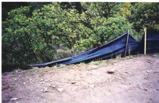
Figure 19: Silt fences around construction sites are rarely constructed properly. This fence provides no water quality protection. Runoff will either flow under or over the filter fabric.
