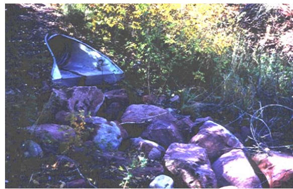
Figure 14: This outfall is properly constructed with a flared end section and riprap outfall.
