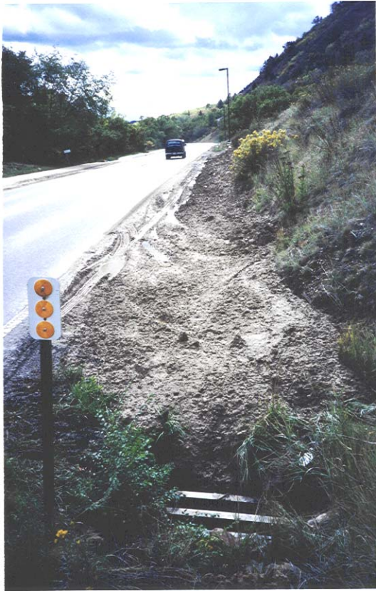
Figure 21: Mud flows from the hillsides currently flow into inlets and are conveyed directly to the rivers where they impact water quality and fill trout spawning beds. This mud flow from Red Mountain has created problems for residents and traffic on Midland Avenue.
