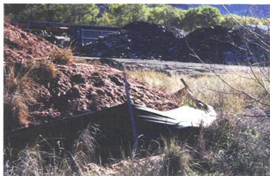
Figure 20: This silt fence is properly anchored and working efficiently to prevent sediment from flowing into the streets and storm drain system.
