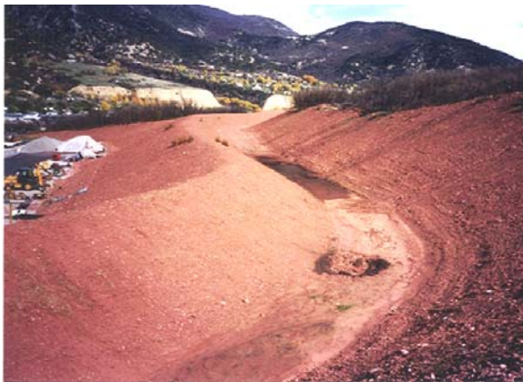
Figure 23: A huge effort was made to protect the Municipal Operations Center from mud flows by constructing this sedimentation basin. The 2002 fires have dramatically increased mud flows from the steep hillsides above the City.
