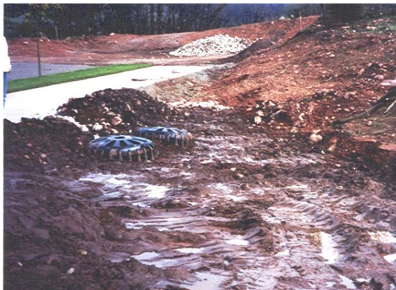
Figure 25: These inlet protection devices are used during construction to keep mud from entering the storm drain system. Filter fabric usually covers the openings. However, as currently installed these devices are providing little water quality protection.
