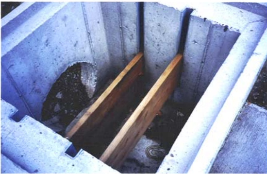
Figure 27: This water quality outlet near the Wastewater Treatment Plant is designed to hold back oils, grease and sediment collected from parking lot runoff. Regular maintenance is necessary to remove accumulated material.
