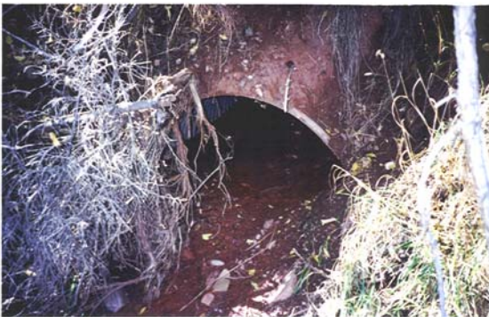
Figure 13: Regular maintenance is required to remove accumulated sediment. This pipe along the south bank of the Colorado River has carried sediment to the river after the recent fires left the hillsides exposed to erosion.
