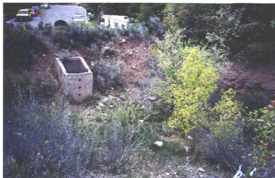
Figure 9: This sedimentation pond, a multi-stage outlet in the Lincolnwood Subdivision, is designed to capture mud and debris and send cleaner runoff to the river, thereby improving water quality.
