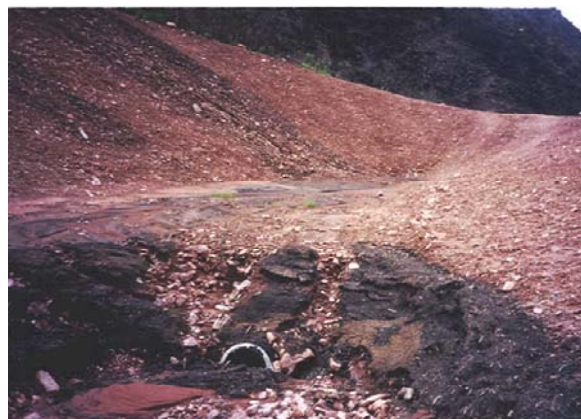
Figure 24: This sedimentation basin behind the Municipal Operations Center protects the building from mud flows, but does little for water quality. The outlet should be retro-fit with a multi-stage outlet to keep sediment from leaving the pond.
