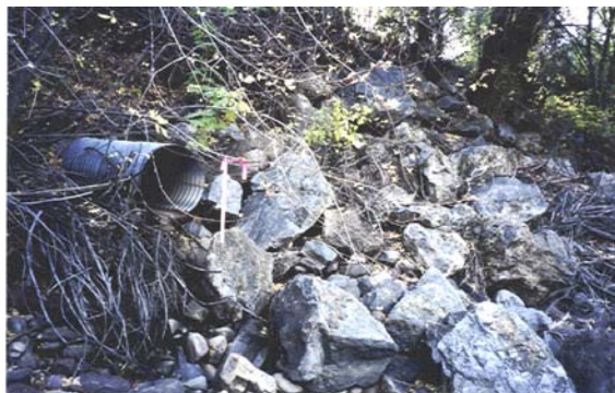
Figure 15: This 24" CMP outfall from the new City Offices into the Colorado River is a potential sampling point for water quality from urban runoff.
