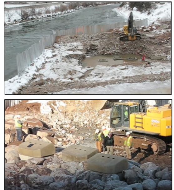
Figure 9. Construction of the Glenwood Springs Whitewater Park during the winter of 2007-2008. In the top photo, a coffer dam diverts the flow of the Colorado River as work is completed on the drained riverbed. In the lower photo, construction crews install wave-generating features, which could qualify as “physical control structures” for purposes of a petition for a RICD water right by the City of Glenwood Springs. (Glenwood Springs Whitewater Park)
