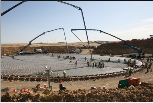
Figure 4. In March of 2009, workers began pouring the foundation for the 10 million gallon Robertsdale Tank, a key component of the Prairie Waters Project. (Aurora Water)
