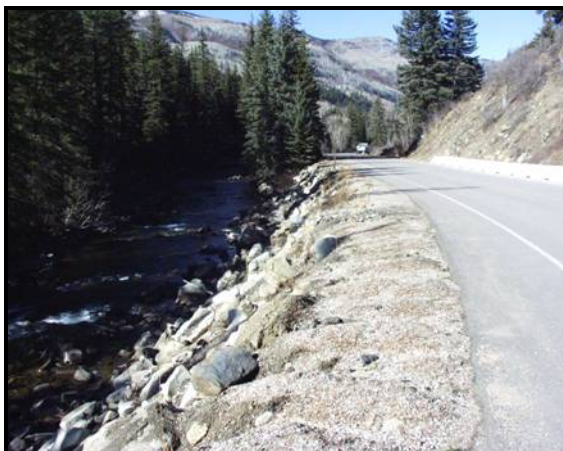
Figure 4.8.13. CR1-2: The roadcut has eliminated streambank stabilizing vegetation, resulting in bank instability, erosion, and stream sedimentation.
