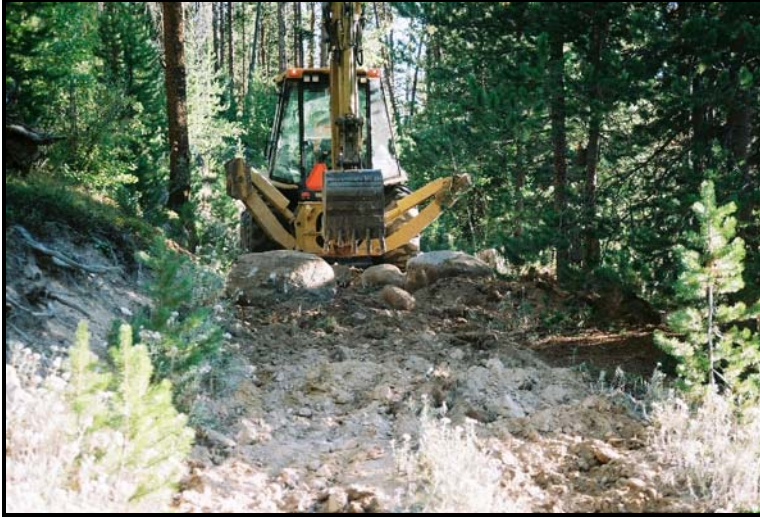
Figure 4.7.15. Decommissioning a non-system road at Sellar Lake, September 2007, (Photo Credit: Mark Lacy).
