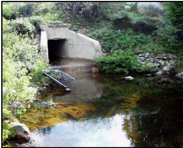
Figure 4.1.23. Upper photo: Lost Man Creek above the dam. Lower photo: Lost Man Creek below the dam. Very little water is left in the stream to maintain the channel or flush sediment from the stream.
