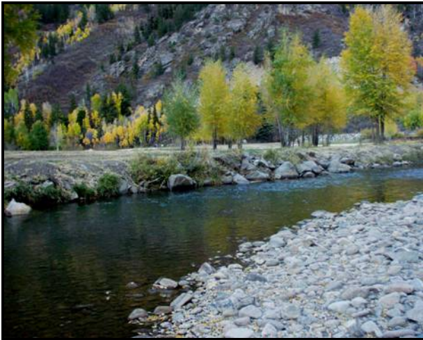
Figure 4.1.22. Removal of native vegetation and bank riprapping has degraded riparian and stream habitat. Fish habitat has consequently been degraded.
