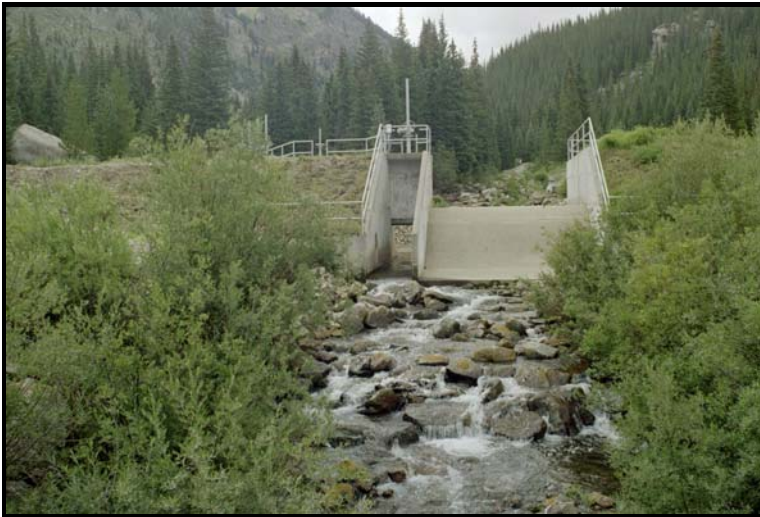
Figure 4.7.9. View of upper and lower ends of Fry-Ark Project diversion structure on Chapman Gulch (August 14, 2006).
