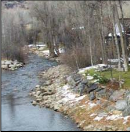
Figure 4.1.19. In this location, riparian vegetation has been removed and replaced with a lawn. Resulting erosion has necessitated bank ripraping.
